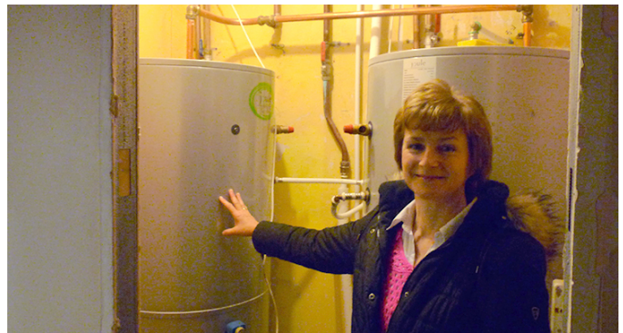
Jenny Kent, proprietor Abbeyleix Manor Hotel, seen here with the hotel's new hot water tanks.
